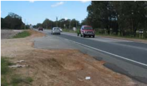
Intersection of Centre Way with Gnangara Rd showing potholes and rough edges.
